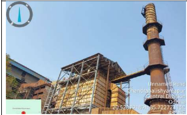
FAP 1x18MVA (Stack & Baghouse)
