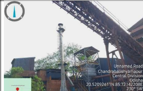
Briquetting transfer points (Stack & Baghouse)
