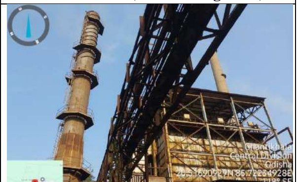
SMS Secondary (Stack & Baghouse)
